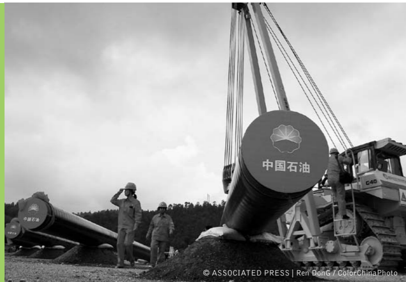
Workers prepare to launch the China section of the Myanmar-China oil and gas pipeline in Anning in southwest China's Yunnan province on September 10, 2010.
